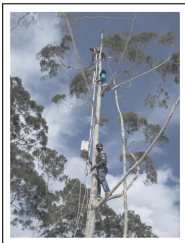
Figure 2. Our BTS installation.
